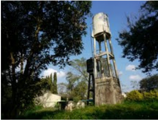
the present water tank
