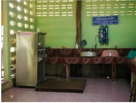
drinking point and nonfunctional filter
