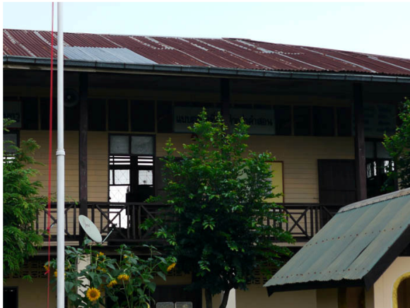
school building with rusted roof
