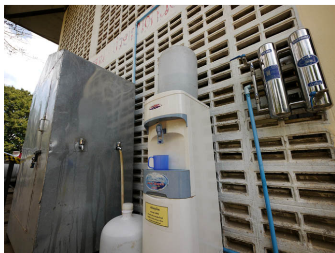
nonfunctional water filter
