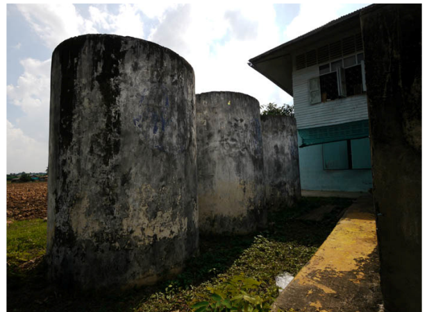
school water tank
