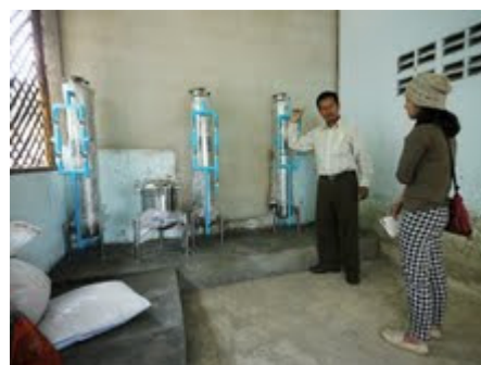
The principal show the new water filter
